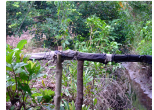
PIPES USED FOR ENTERPRISE DELIVERED RURAL WATER SUPPLY IN THE MEKONG REGION OF VIETNAM
