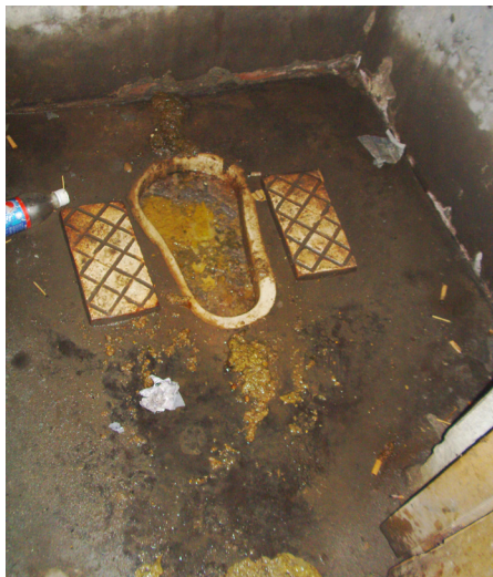
Filled up pit latrine Syedpur Village, Bangladesh. Credit: Suzanne Hanchett
