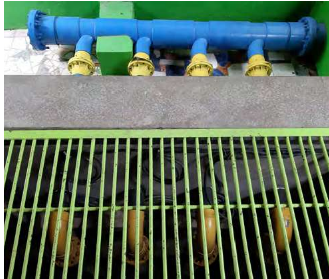
Bar screen with submersible pump
