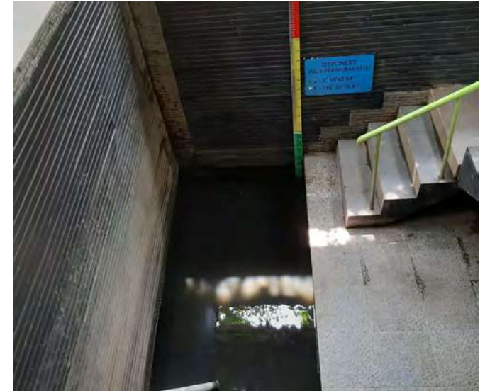
Raw sewage pump station
