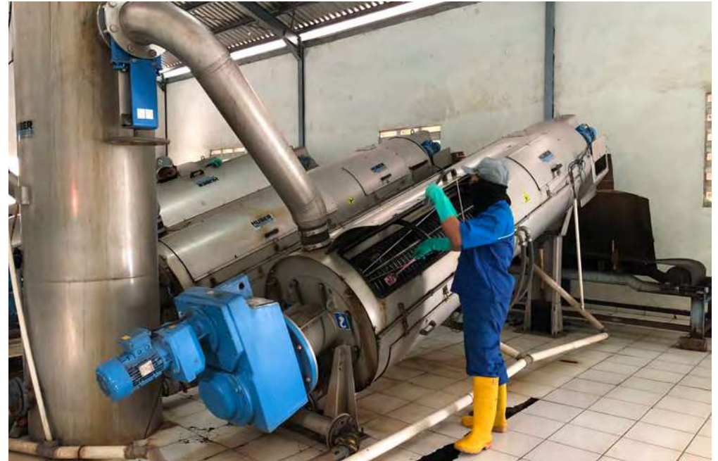
A Huber screw press unit in operation
