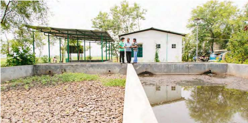
Sludge drying beds at the Kushtia FSTP
