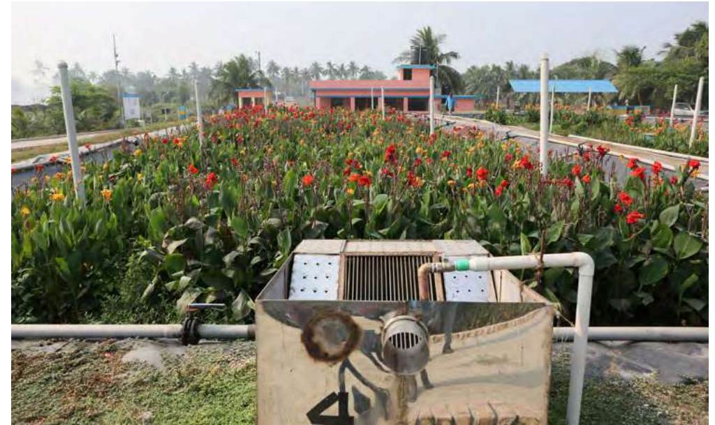
Manual bar screen to remove garbage from sludge discharging into vertical flow constructed wetland
