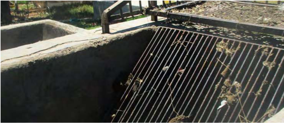
Chazanga FSTP grit separation at influent discharge point
