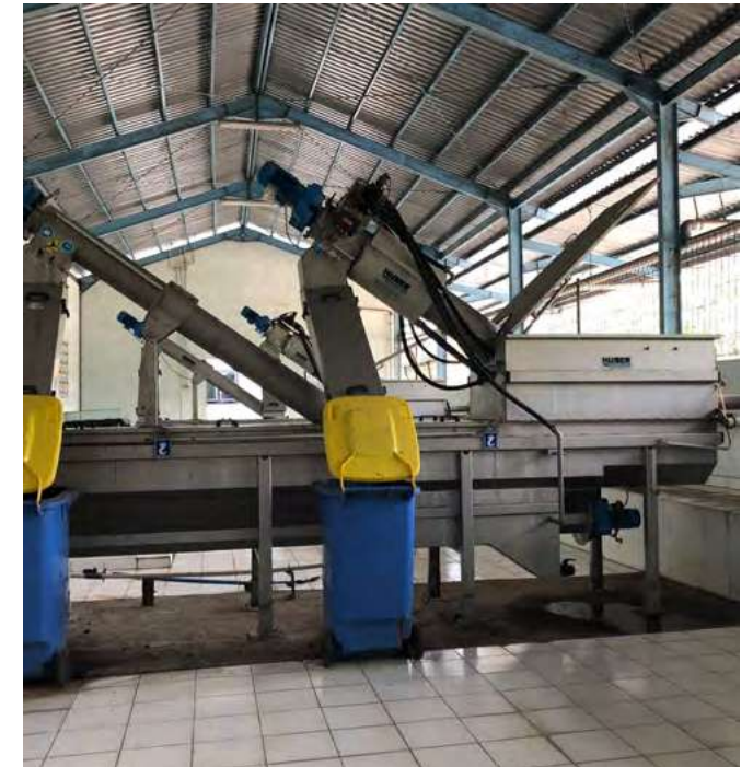
Mechanical sludge screening using Huber acceptance plant
