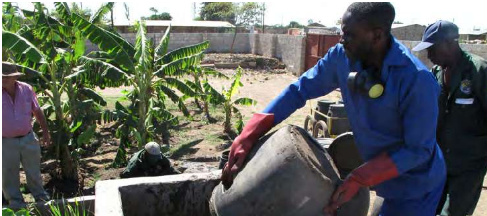
Kanyama FSTP worker emptying sludge
