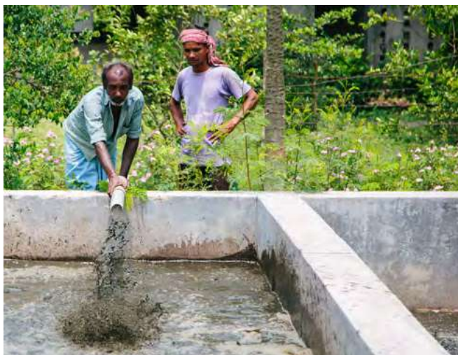
Discharging sludge into drying beds
