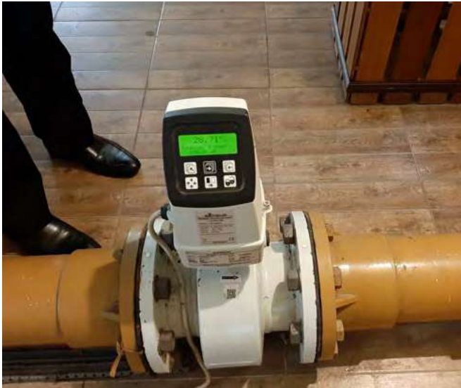
Inlet automatic flowmeter
