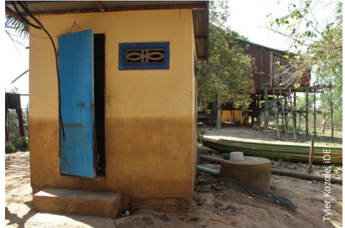
An unusual flood event in a rural village in Kampong Thom Province, Cambodia leaves a visible high-water mark on the latrine shelter. The flood water inundated the latrine pit, causing the system to overflow and become dysfunctional.
