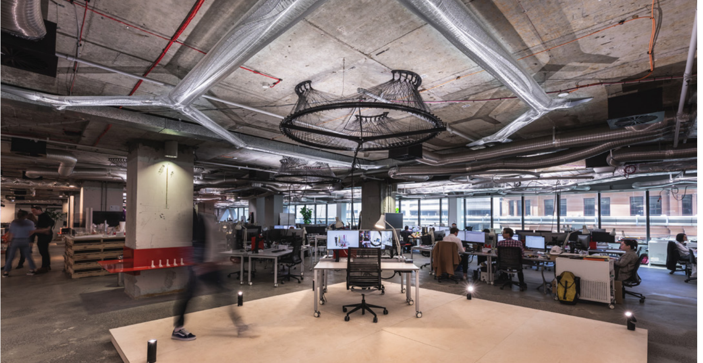
SR2 installed in the BVN office space in Sydney
