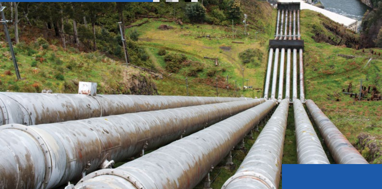
Penstocks feeding the Tarraleah Power Station, a pumped-storage hydroelectric power station in Tasmania, Australia.
