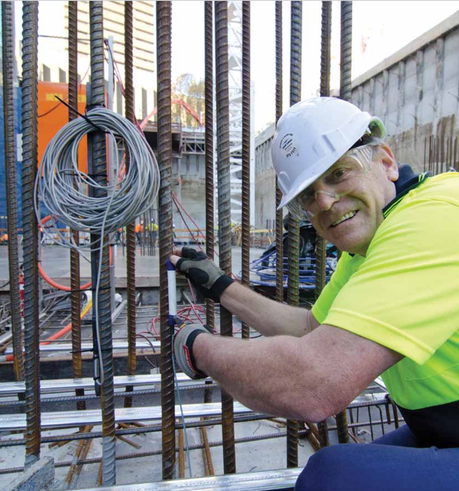
Ray Clout, manager of research laboratories for the Faculty of Engineering and Information Technology, installing sensors into the Broadway Building.
